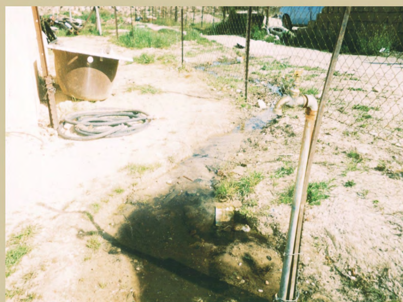
Figure 2. In the most severe instance a leak accounted for almost 350kl water consumed per month
