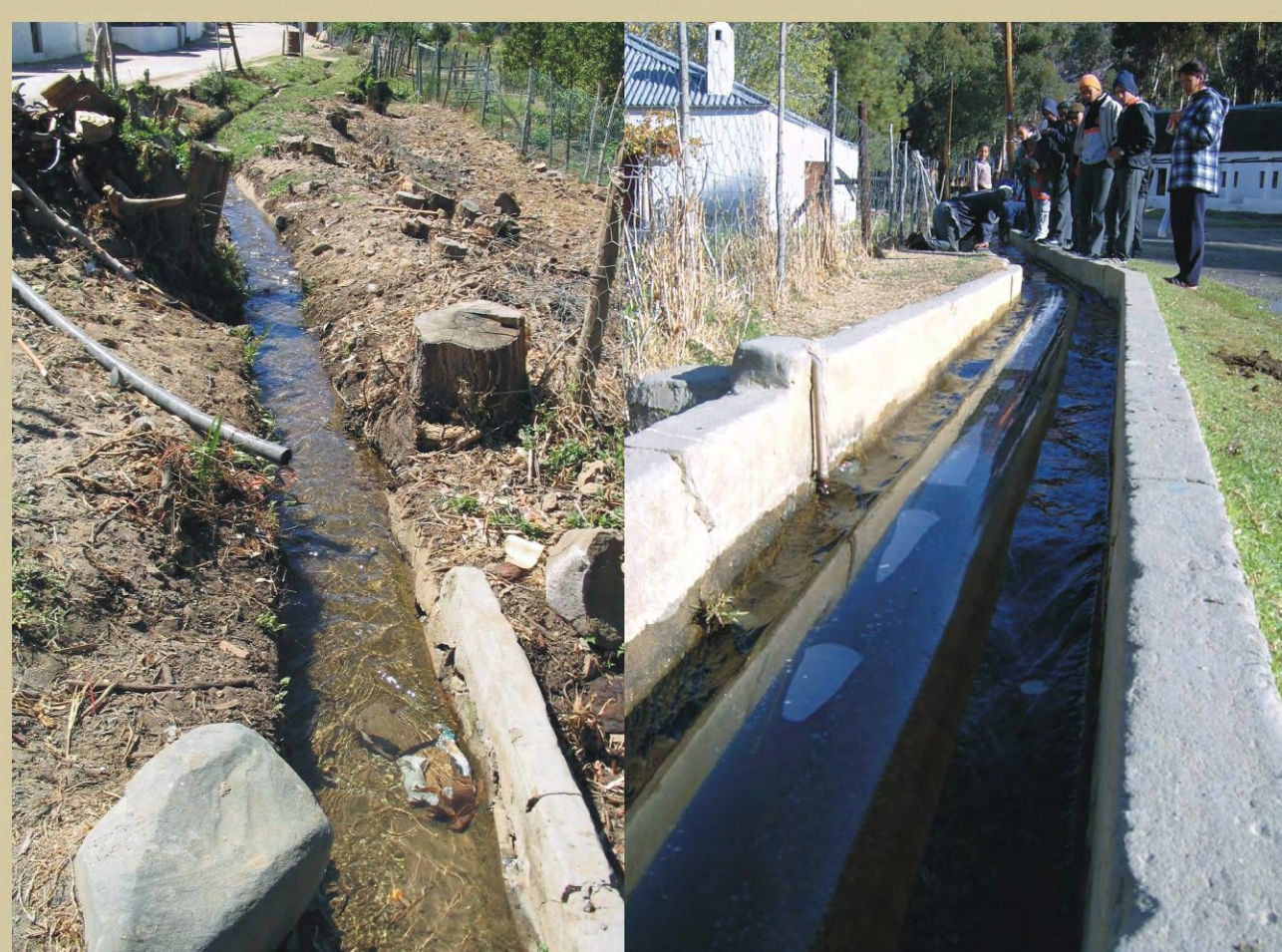
Figure 4. In Wupperthal water loss is experienced due to many cracks and seepage along the canal. The micro-project uses a cost effective, lay-flat pipe to conserve water while creating greater awareness.
