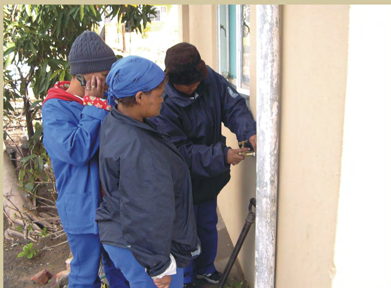
Figure 4. The Clanwilliam leak repair team hard at work replacing a leaking tap.
