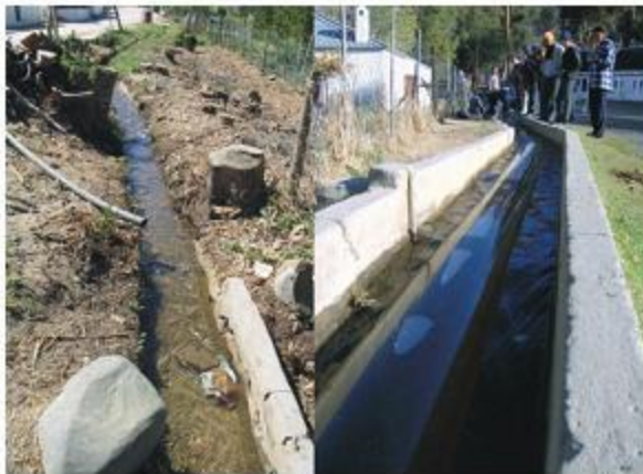
In Wupperthal water loss is experienced due to many cracks and seepage along the canal. The micro-project uses a cost effective, lay-flat pipe to conserve water while creating greater awareness.
