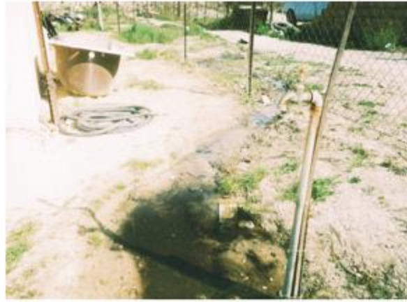
In the most severe instance a leak accounted for almost 350kl water consumed per month
