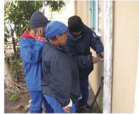
The ladies of the Clanwilliam leak repair team hard at work replacing a leaking tap.
